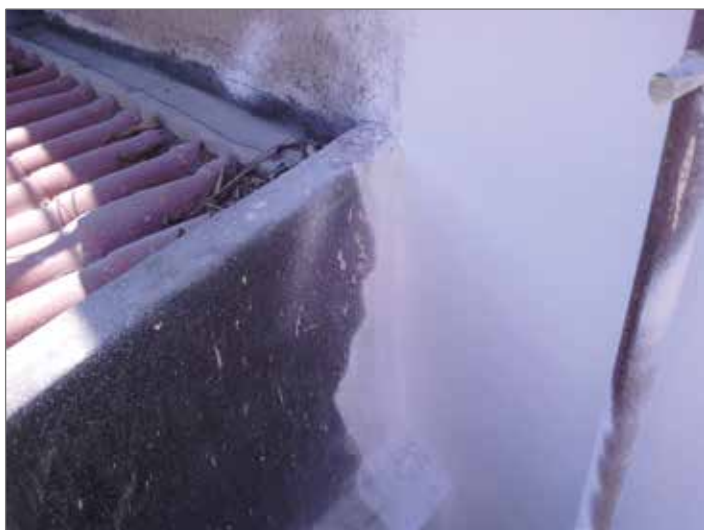
Img 9. Comparison of treated and untreated surface area on the south side of the building, photographic survey.
