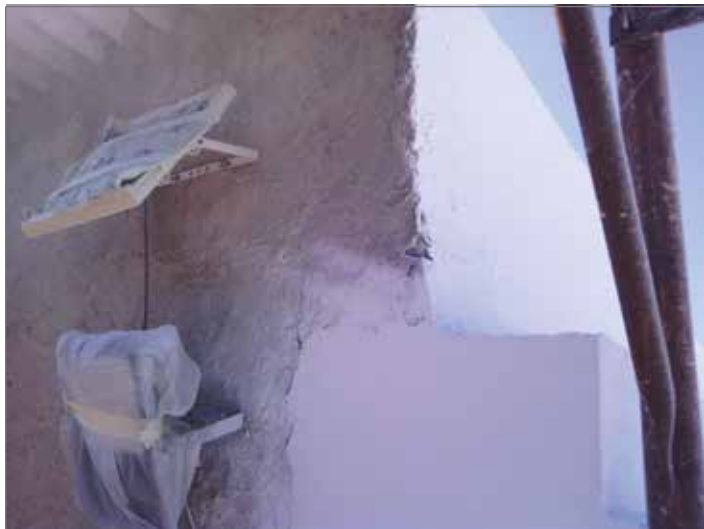
Img 7. South wall surface of adjacent building (untreated) and East wall (treated building) photographic survey.
